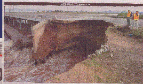
Workers check out damage to Alma School Road due to erosion of the Salt River bridge's approach. The bridge, on the Salt River Reservation north of the Loop 202, has not suffered damage and is not in jeopardy but is closed.
